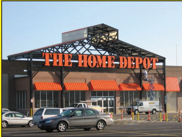
Left: The 145,000 SF Cleveland Home Depot was built at the site of a former steel foundry in downtown Cleveland, and is part of a new retail development called Steelyard Commons. The project began last June with the installation of 914 steel pile foundations, 72 feet deep into the bedrock, and finished with a new home improvement warehouse for the residents of Cleveland.
